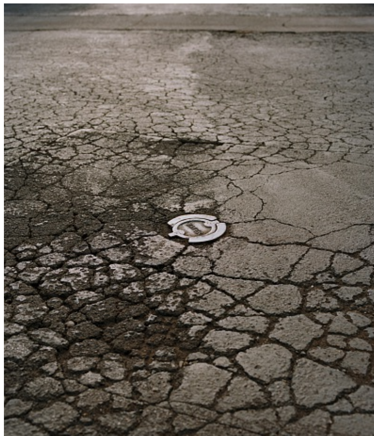
Cracked asphalt on the roads at Shadowbrook
